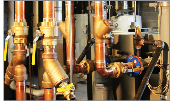
New Copper Water Connections
